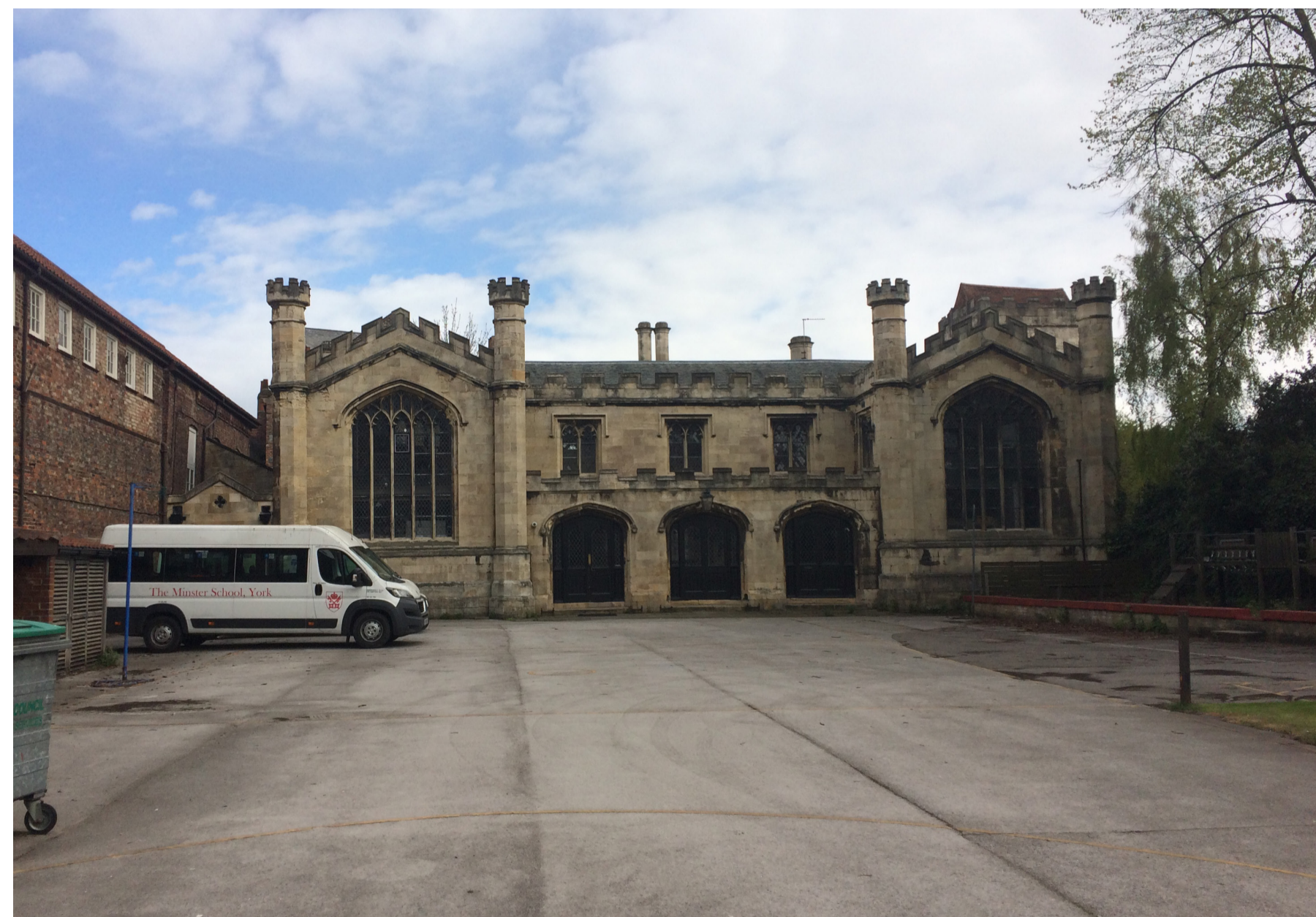
The former song school is vacant and in need of extensive and ongoing repairs
