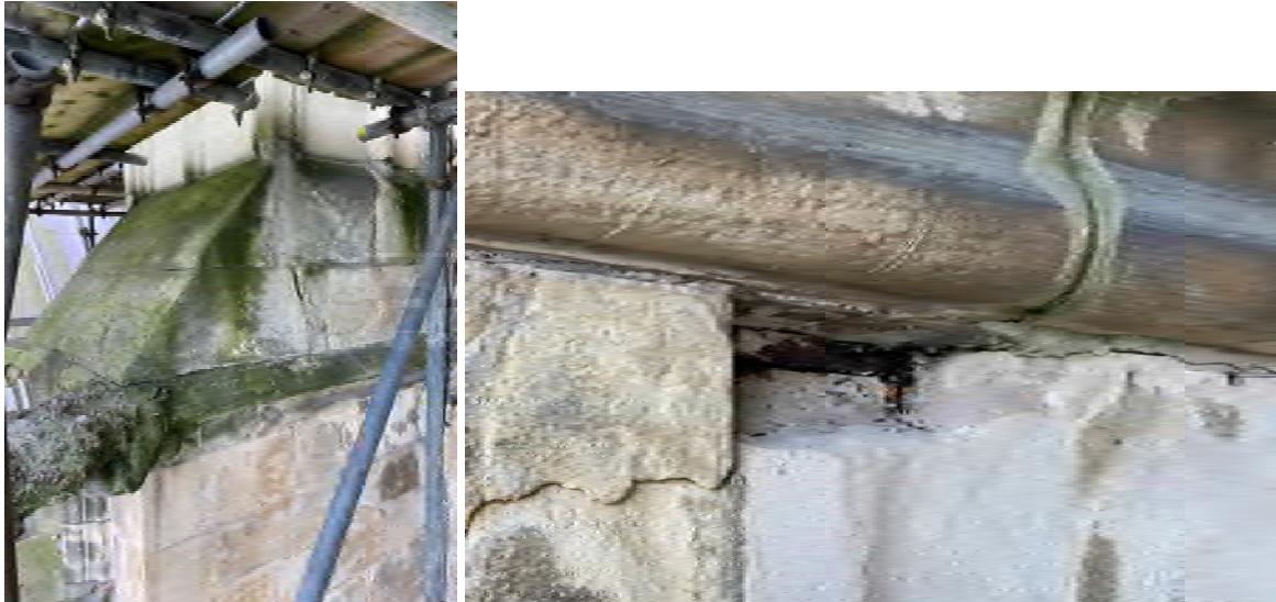
Left: cracking and rust-jacking has now been noted in the root of the pinnacle both sides of the upper buttress weathering. Right: embedded iron revealed behind spalled stone.
