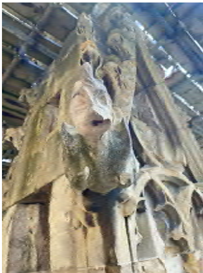
Example of a ‘relict’ grotesque which will be re-carved. Where appropriate features and forms are taken from surviving carvings as the root for new work.
