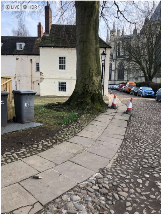
Plate 3. Section of paving to be replaced
