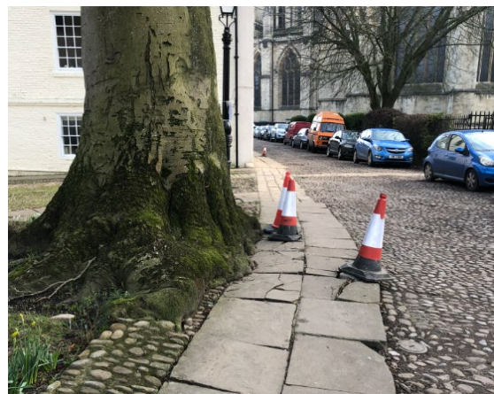
Plate 2. Area of paving lifted by tree roots.
