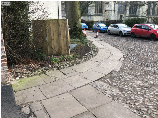
Plate 5. Extent of flags to be replaced
